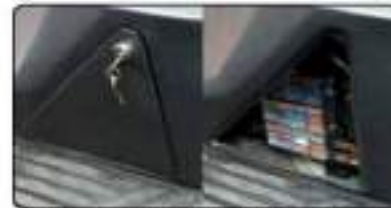
New fuse panel providing service accessibility
